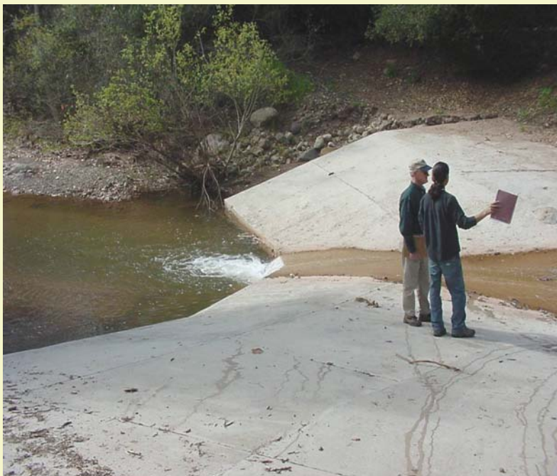
Low water crossing creating barrier for steelhead trout migration
