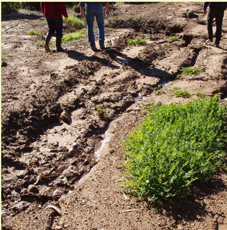
Gully erosion along road caused by concentrated flow from stormwater runoff
